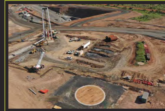
The construction of Ironbark No.1 is progressing well. The all-weather surface roads are in the process of being constructed and the drifts are 2 months from reaching the seam. An exciting milestone up ahead for the team.
